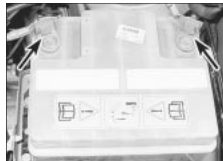
2.3 Battery lead terminals (arrowed)
