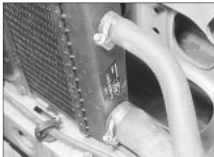
5.2b . . . the bottom hose and expansion tank hose
